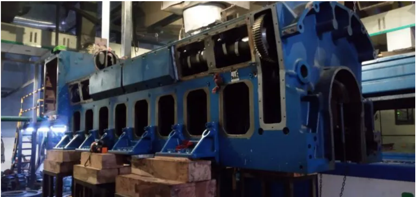
MWM TCG 2032 V16 gas engine during the E70 general overhaul. (Photograph: Hindustan Syringes & Medical Devices Ltd.)
